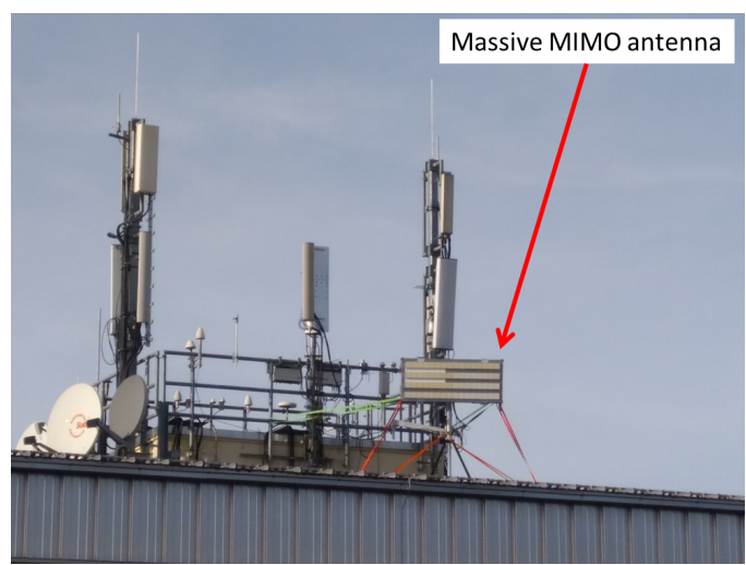
Fig. 3. Massive MIMO antenna of 64 antenna elements (4 lines and 16 columns of antenna elements) on the roof of a building of Nokia Bell Labs campus in Stuttgart, Germany.
